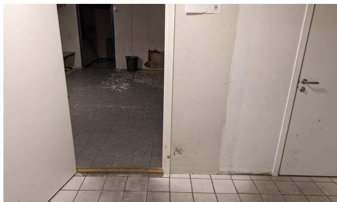
Garderoberne var veldig klar for totalrenovering.
